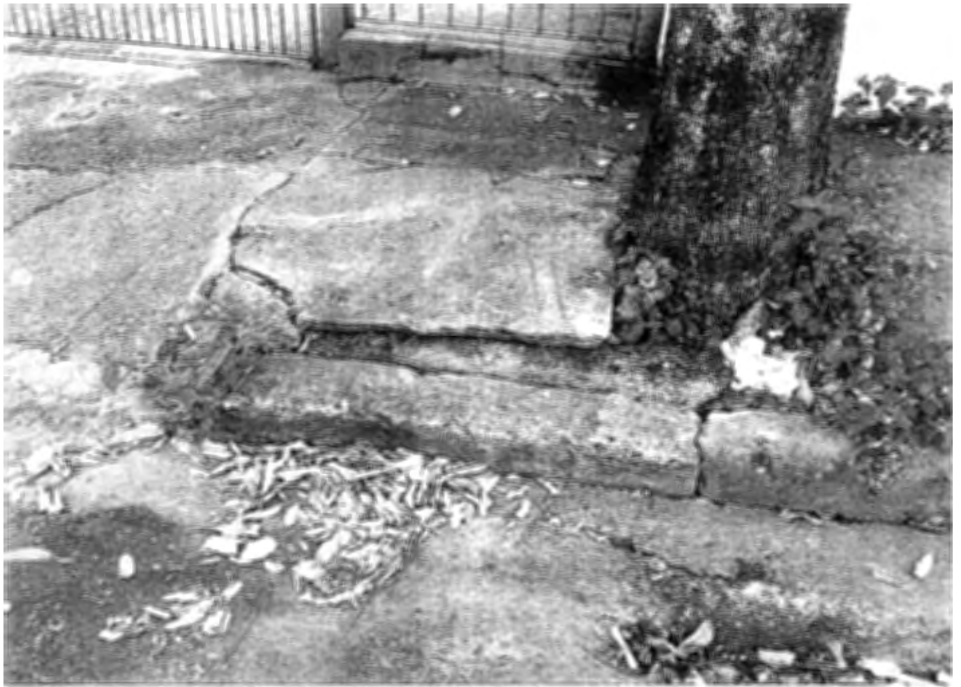
Figure 1: Stone paving and debris.
